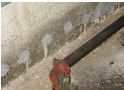
Figure 3. Post Injection Patch
