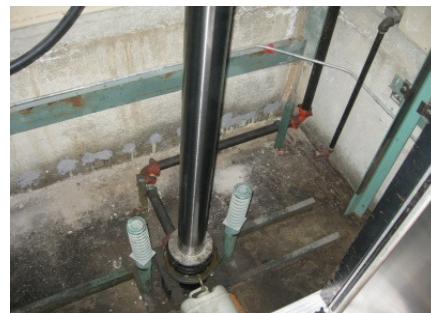
Figure 4. Dry Elevator Pit
